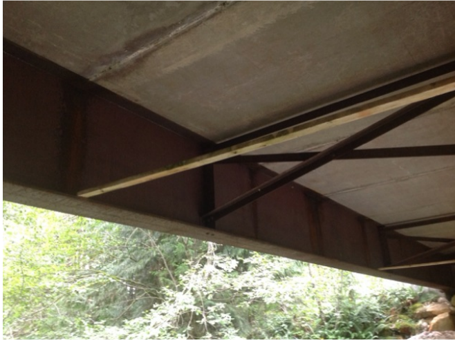
deck joints from below - note corrosion on girders in these locations
