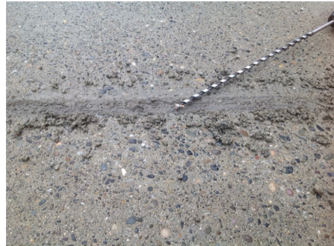
deck joints not filled right to surface - 10mm below
